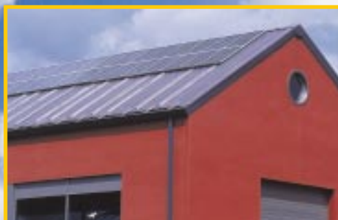
Photovoltaikanlagen in Ettelbrück und in Noerdange*
